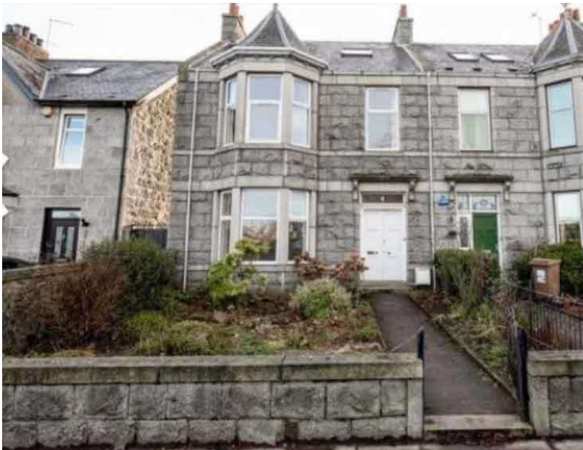
Photo 1: Demonstrating the front of the Appellant's property along with the dilapidated state of its garden following the passing of the previous owner.
