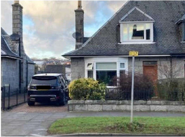
Photo 5: Demonstrating that 58 Cromwell Road has removed a section of low-lying granite wall in order to create a car park to the front of the property.
