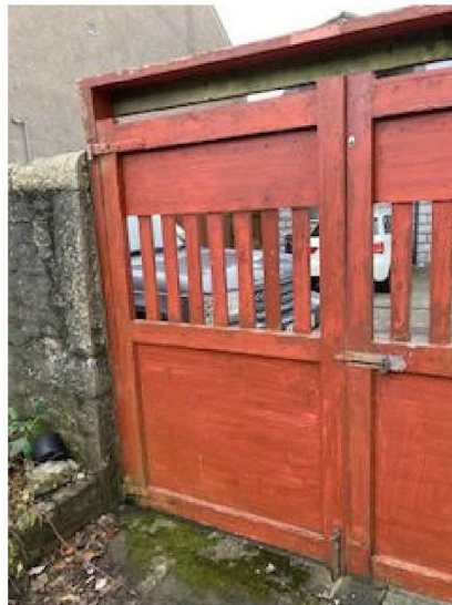
Photo 28: Demonstrating that it would be unreasonably difficult to reverse out of the Appellant's rear gate when another car is legally parked in the space, such as this grey range rover.
